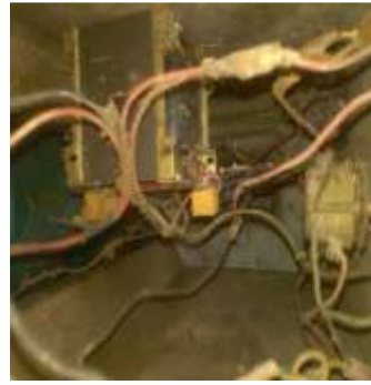
Figure 6: The wiring of Electromagnetic Separator
