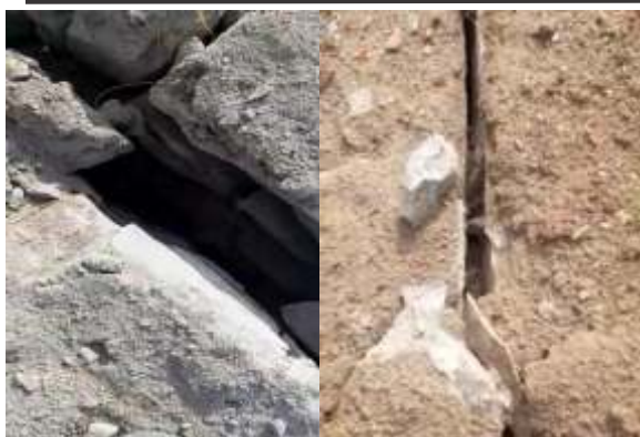
Fig. 3.3: Cracks due to vibration from blasting (at Zeberced quarry limited)
